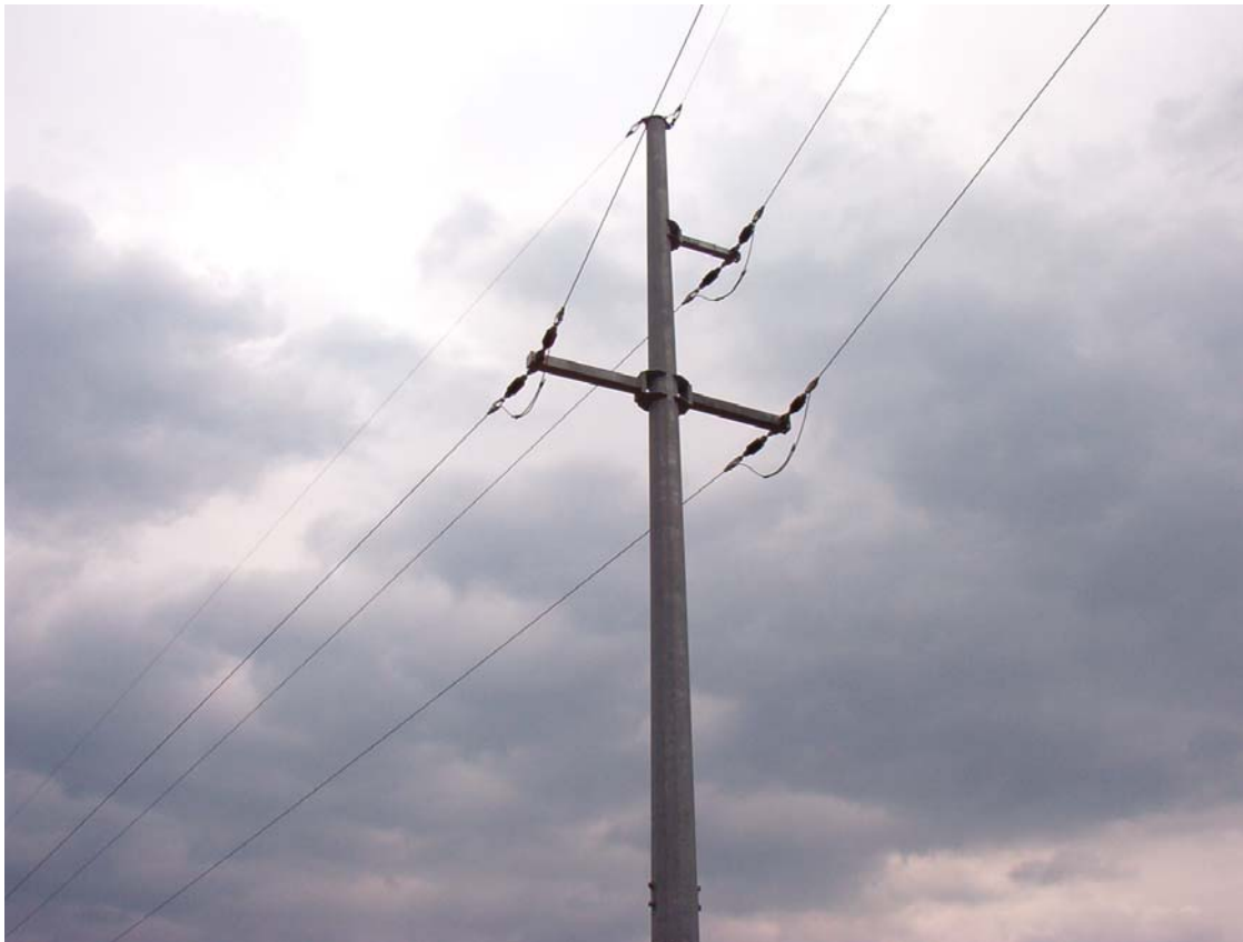
Hollow steel pole in the role of angle support of single circuit 35 kV overhead line with the protection conductor
