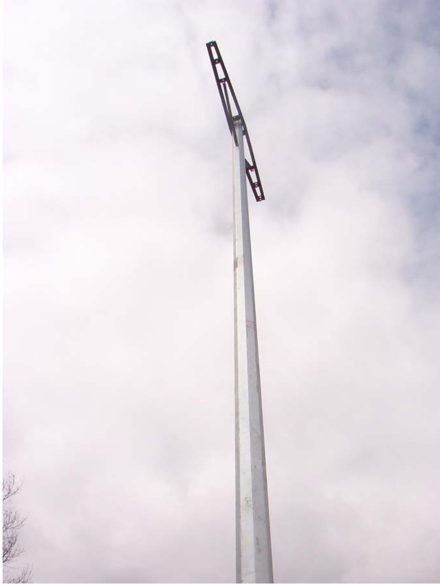
Hollow steel pole playing the role of intermediate support of 10 kV single circuit overhead line prepared for further installation (insulators and conductors)
